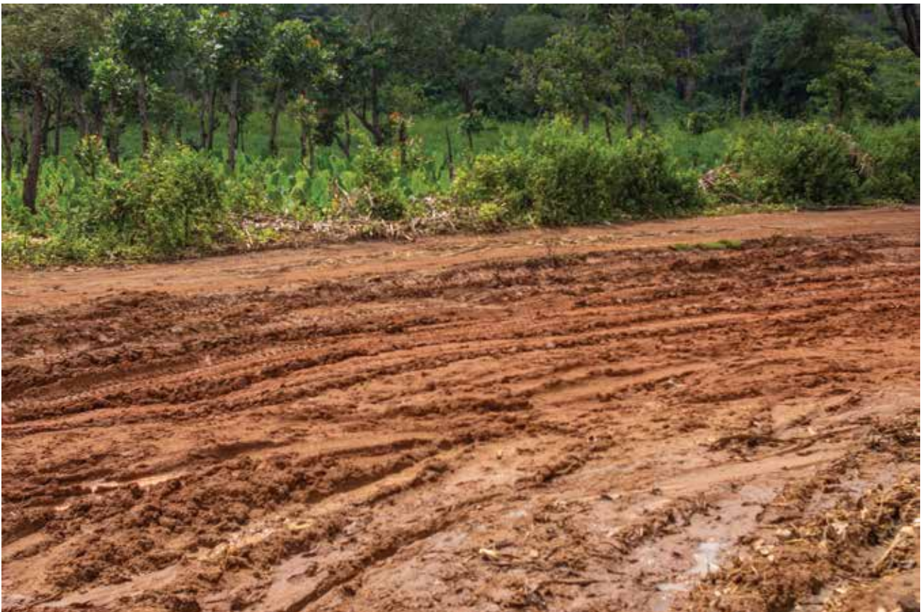
State of the road leading to Kuzhako Community
