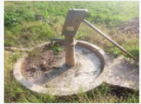
Non functional hand pump borehole in Kuzhako
