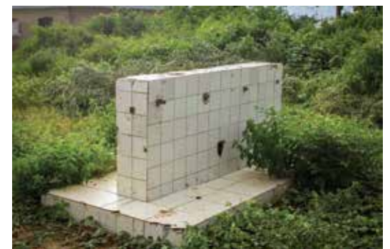
Non functional borehole
